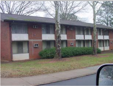
Exterior of Building E, to be remodeled in 2007. Note the condition of the roof and the exterior A/C units.
